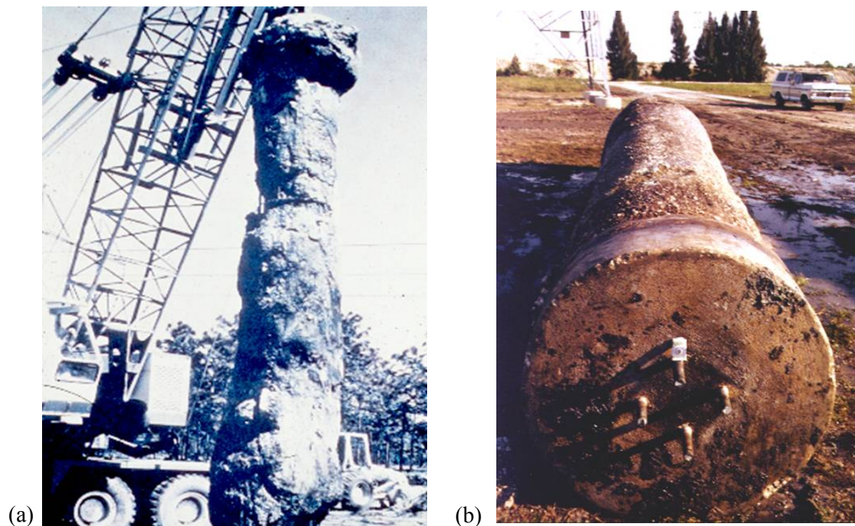
Figure 9-57. Photographs of exhumed shafts (a) shaft where excavation was not adequately cleaned, (b) shaft where excavation was properly cleaned (FHWA, 2002d).
